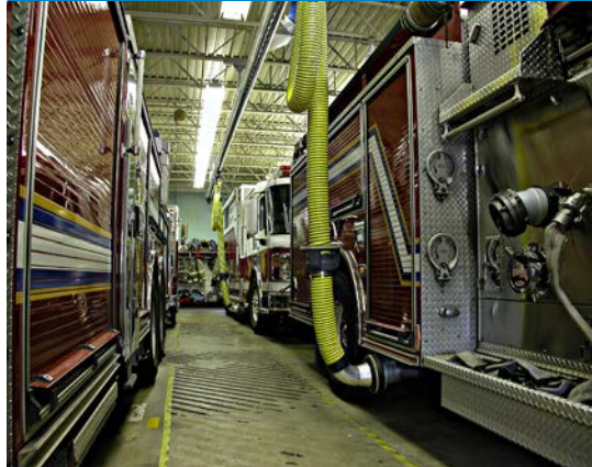
Figure 6.12 — A typical source capture exhaust filtration system.
